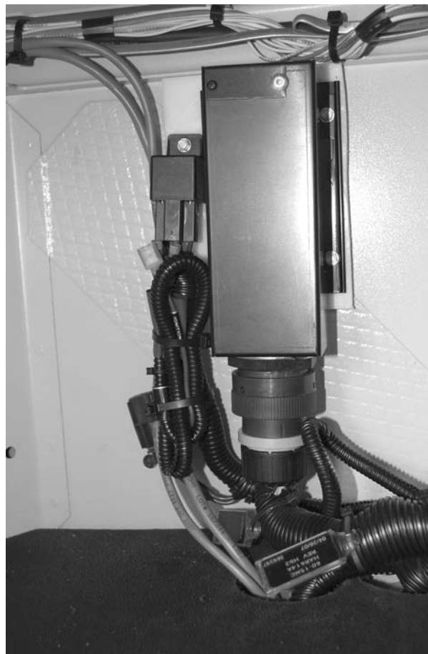
Figure 7 – Regulator mounted inside truck
